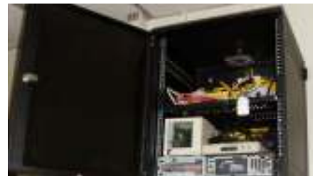
Equipment at GPS Base Station
